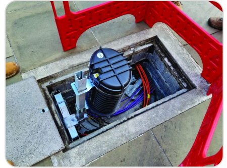
— DEPLOYED EQUIPMENT CARRYING ITS OWN VERIFIABLE RECORD
