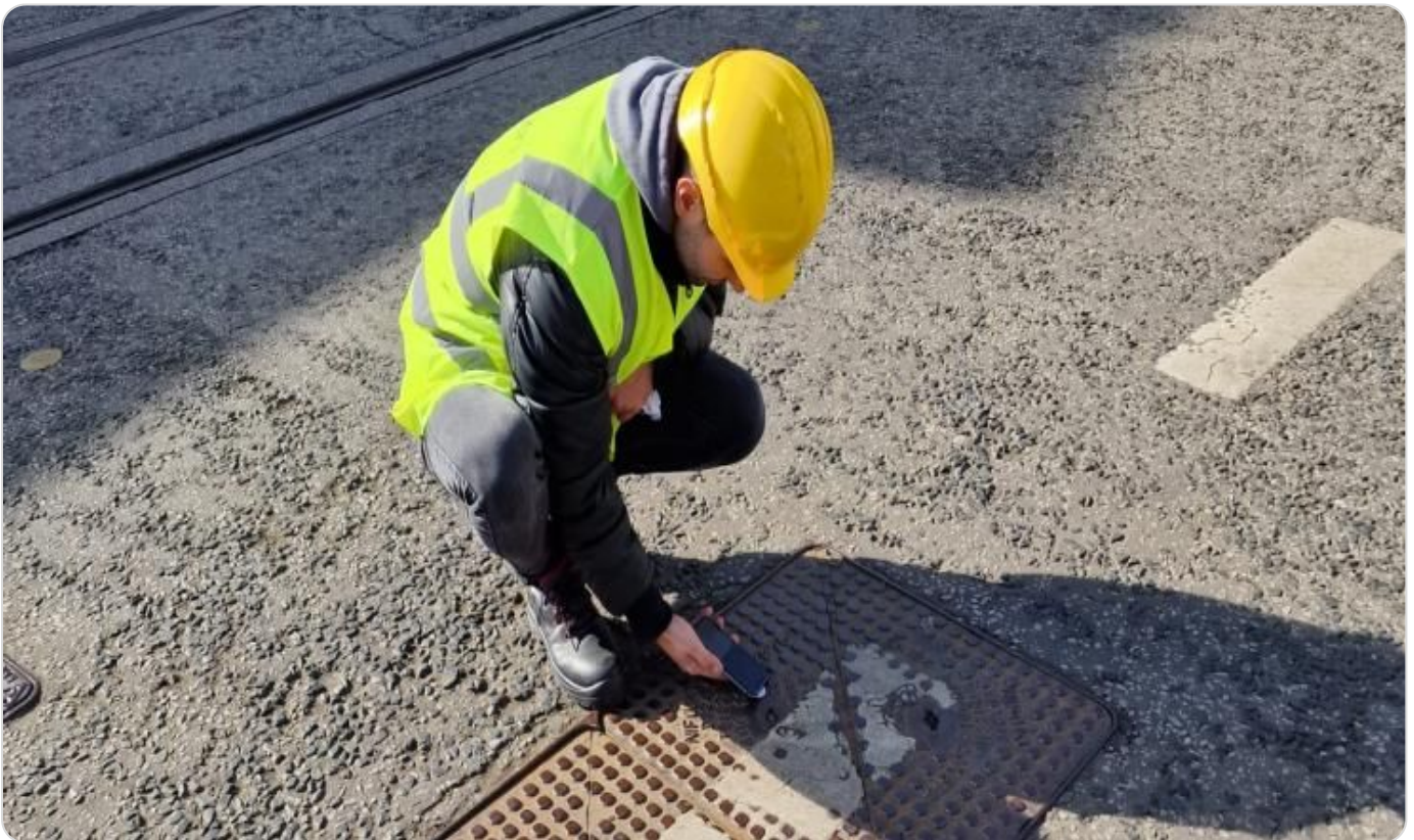
SCANNING A LOC TAG ON A STREET VAULT
